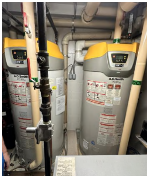
Figure 8: A.O. Smith Water Heaters for Arena-DHW Heating
